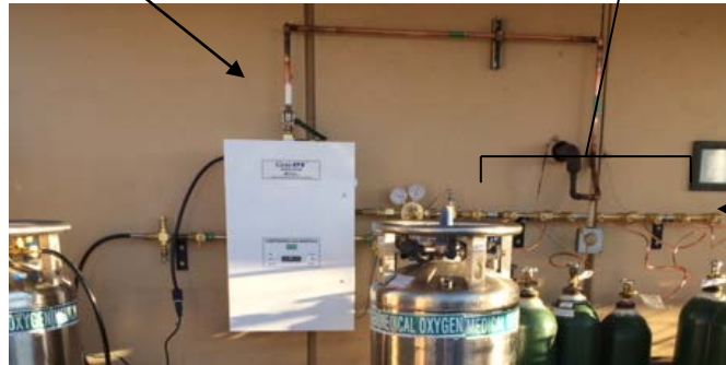
Emergency reserve low pressure transducer (14-3001)
